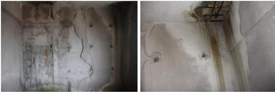
Fig. 8. Example of some defects in Building C.
