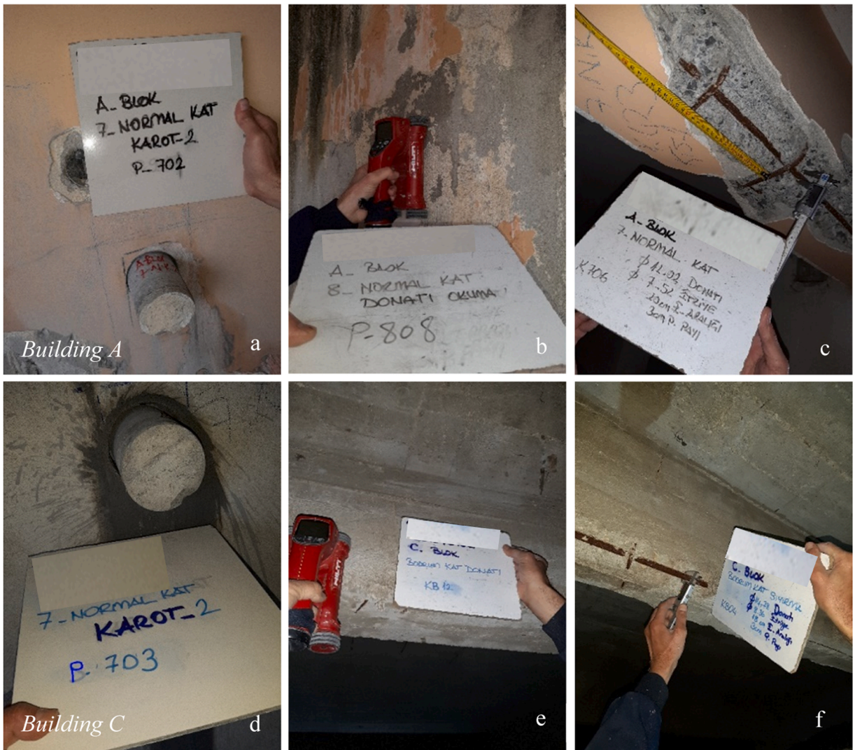
Fig. 9. Core sampling and rebar detection on Building A (a-c) and Building C (d-f).
