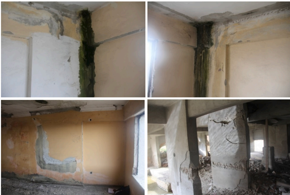
Fig. 5. Example of some defects in Building A.
